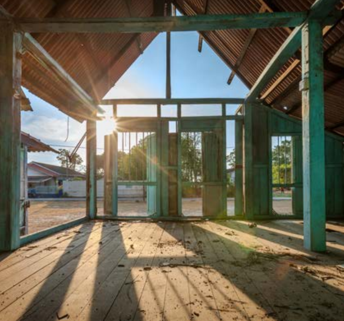
The house today, left vacant and in a state of deterioration.
